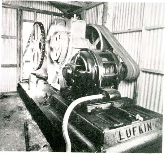
Inside motor house. There is ample room to take off or put on belts on V drive not evident in picture.
