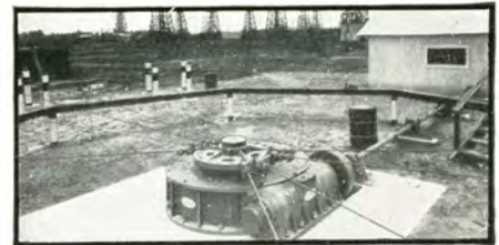
Typical Lufkin Central Power Installation
