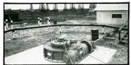
Typical Lufkin Central Power Installation
