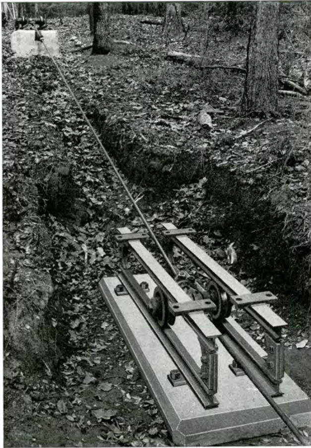
FIGURE 81 Lufkin Roller hold-down in structural frame. Note roller hold-up in distance
