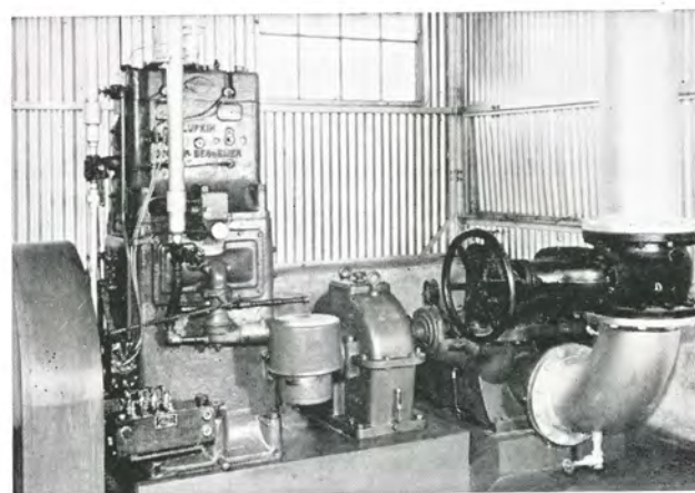
FIGURE 83 Lufkin S105 Reducer driving centrifugal pump in salt water disposal plant. Driven by Lufkin Engine.
