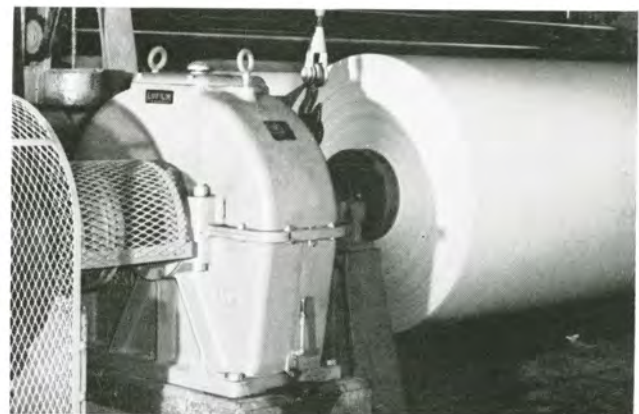
FIGURE 85 Lufkin S189 Single Reduction Herringbone Reducer Driving Rewind Machine at Newsprint Mill.
